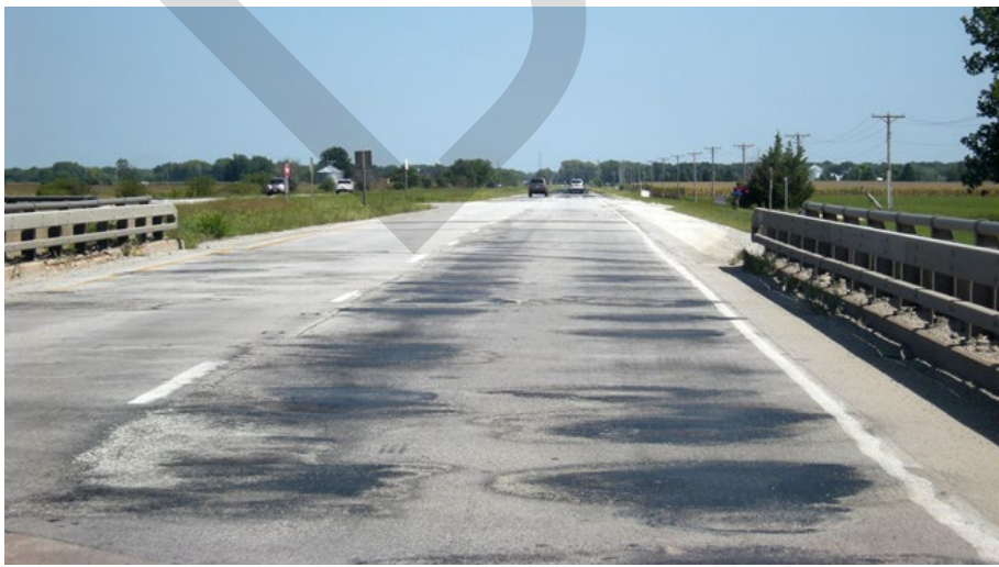
IL-17 Bridges over Baker Creek were in poor condition prior to replacement work in 2019/2020.
