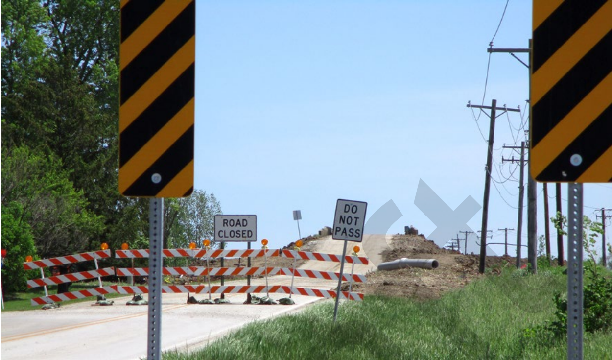
The closure of St. George Road during the bridge replacement over Interstate 57.
